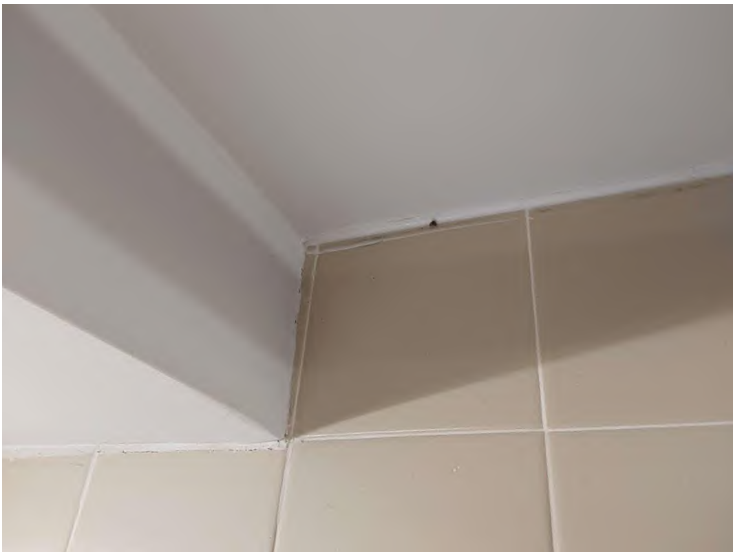
PCB, P0002(No), CAULKING, White caulking along walls, Men's Washroom - C2126 (Location #: 403)
