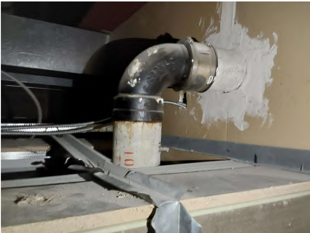
V9000 (Confirmed Asbestos), Piping, Drain, Cement Product, Men's Washroom - B3174 (Location #: 191) Near ceiling hatch
