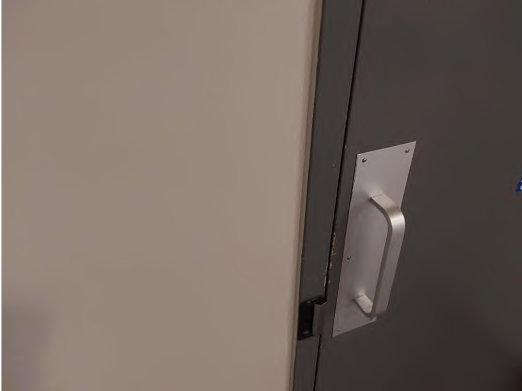
PCB, P0003(No), CAULKING, Beige caulking on door frame, Men's Washroom - B3174 (Location #: 191)
