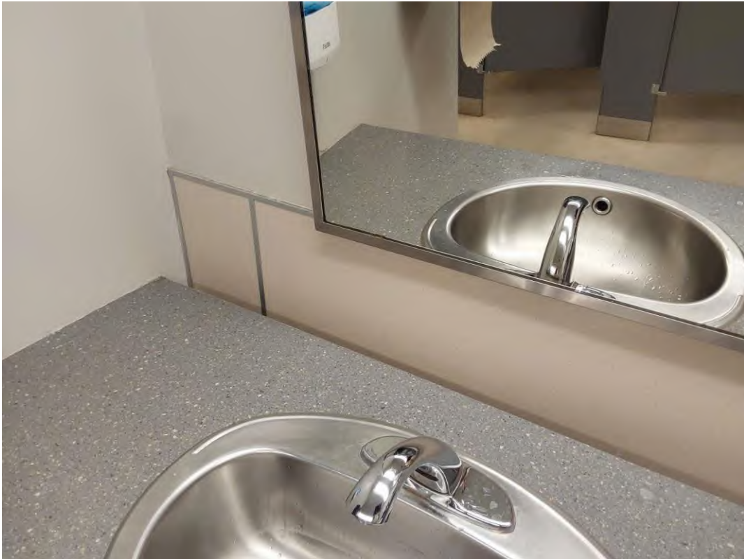
Wall, Plastic, Women's Washroom - B3170 (Location #: 190) Plastic board, adhered with drywall compound and caulking
