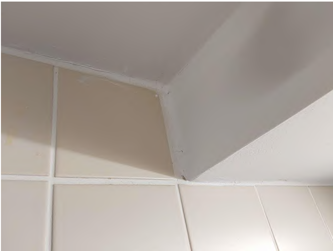
S0075A (None), White caulking along walls, Wall, Caulking, Women's Washroom - C2128 (Location #: 404)
