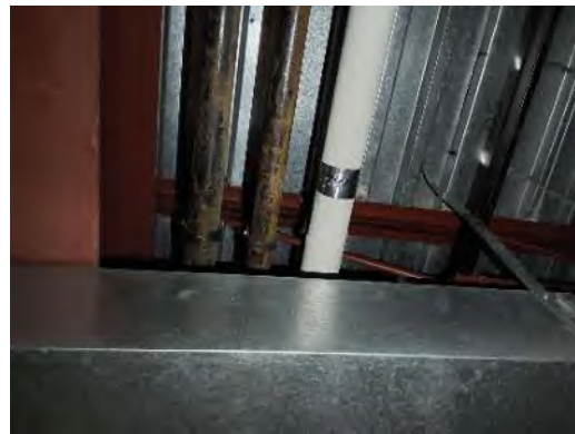
Pipe insulated with fibreglass in the Men's Washroom – B3174 (Loc. 191)
