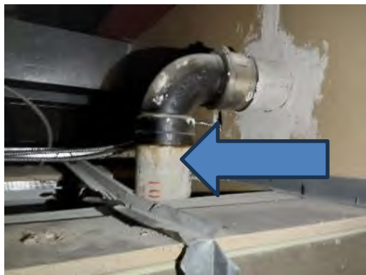
Cement pipe (Transite) in the Men's Washroom – B3174 (Loc. 191)
