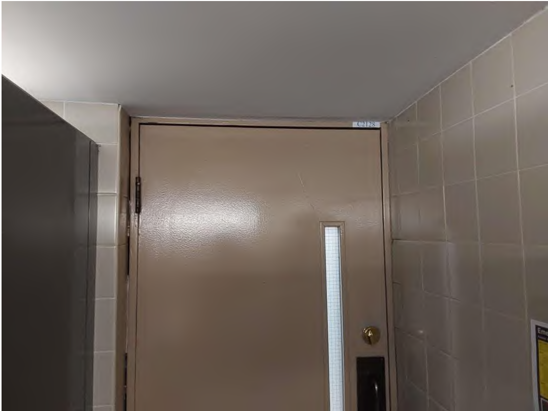
L0006(Lead, None), Beige paint on door, Wall, Men's Washroom - C2126 (Location #: 403)
