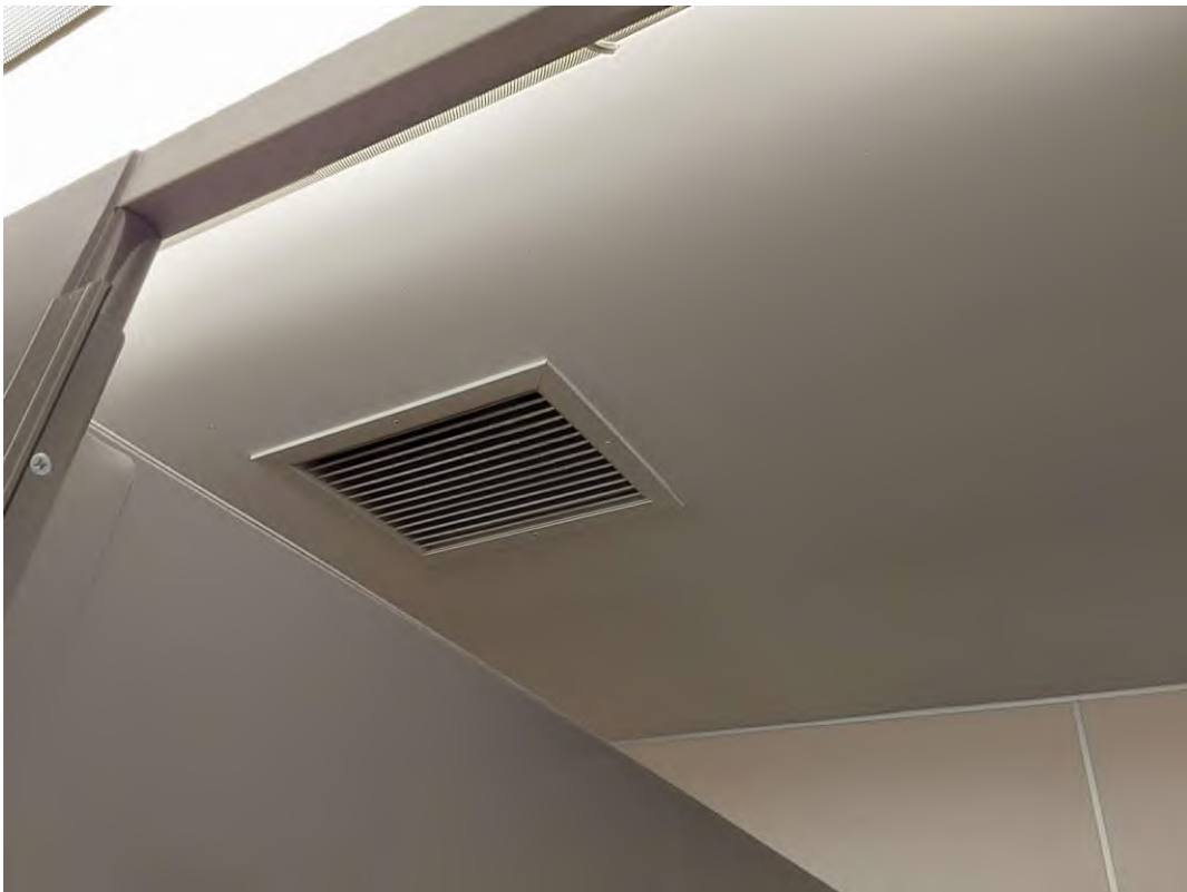
S0077A (None), Drywall on ceiling, Ceiling, Drywall and joint compound, Women's Washroom - B3170 (Location #: 190)
