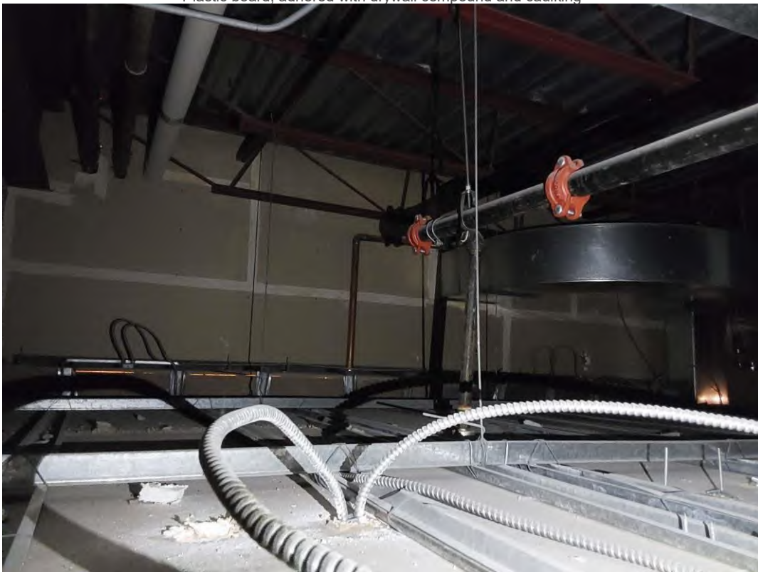
Piping, Not Insulated, Men's Washroom - B3174 (Location #: 191)
