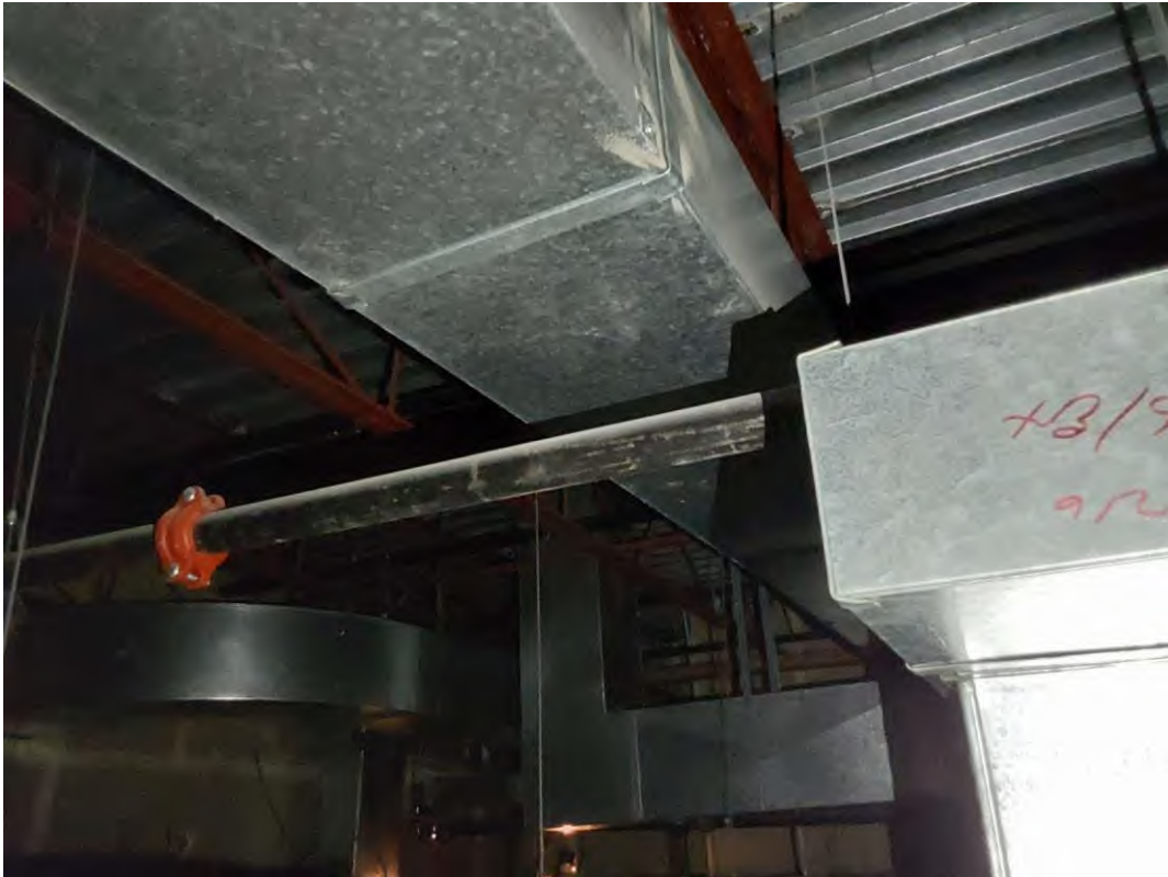
Duct, Not Insulated, Men's Washroom - B3174 (Location #: 191)
