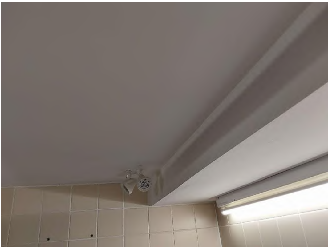
L0005(Lead, None), White paint on drywall, Ceiling, Men's Washroom - C2126 (Location #: 403)
