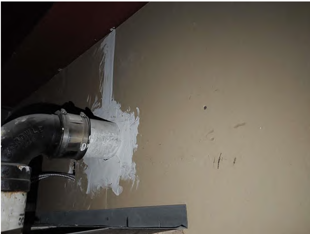
S0078B (None), Wall, Drywall and joint compound, Men's Washroom - B3174 (Location #: 191)
