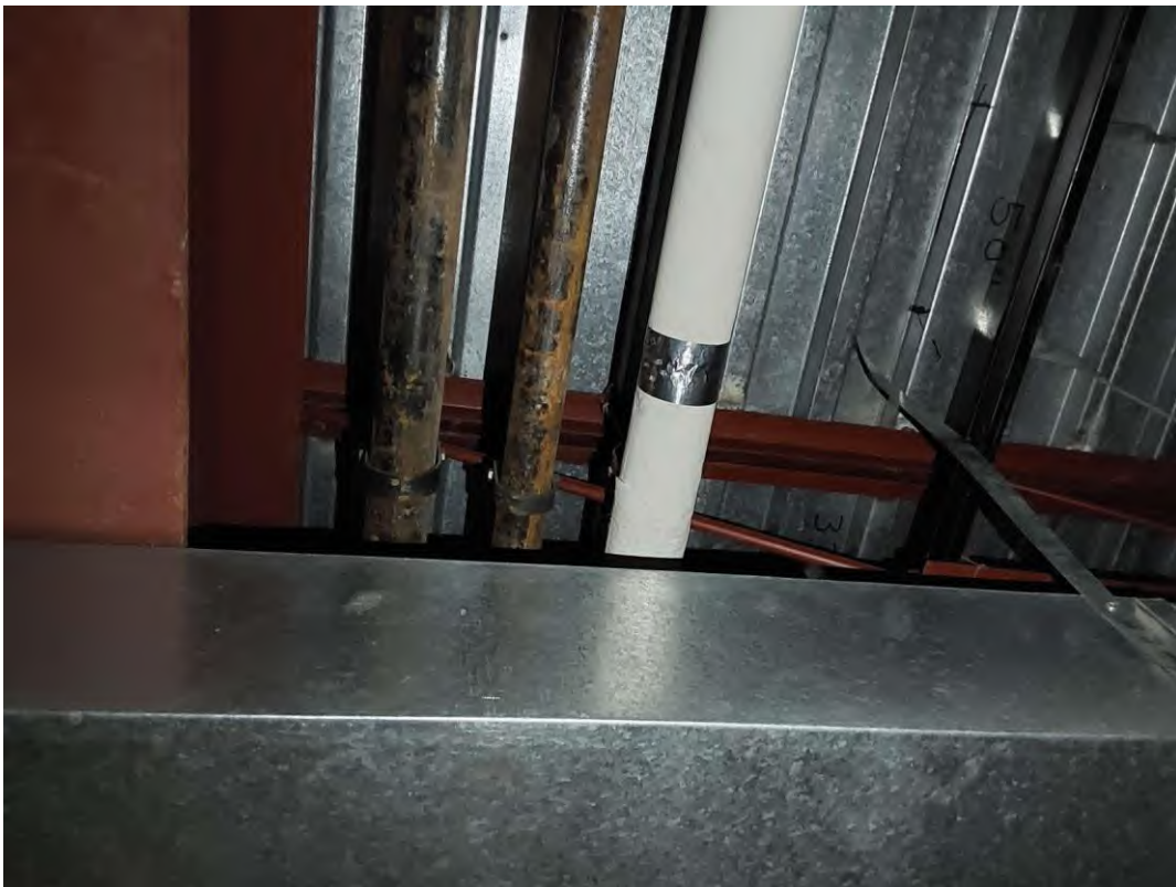
Piping, Fibreglass, Men's Washroom - B3174 (Location #: 191)
