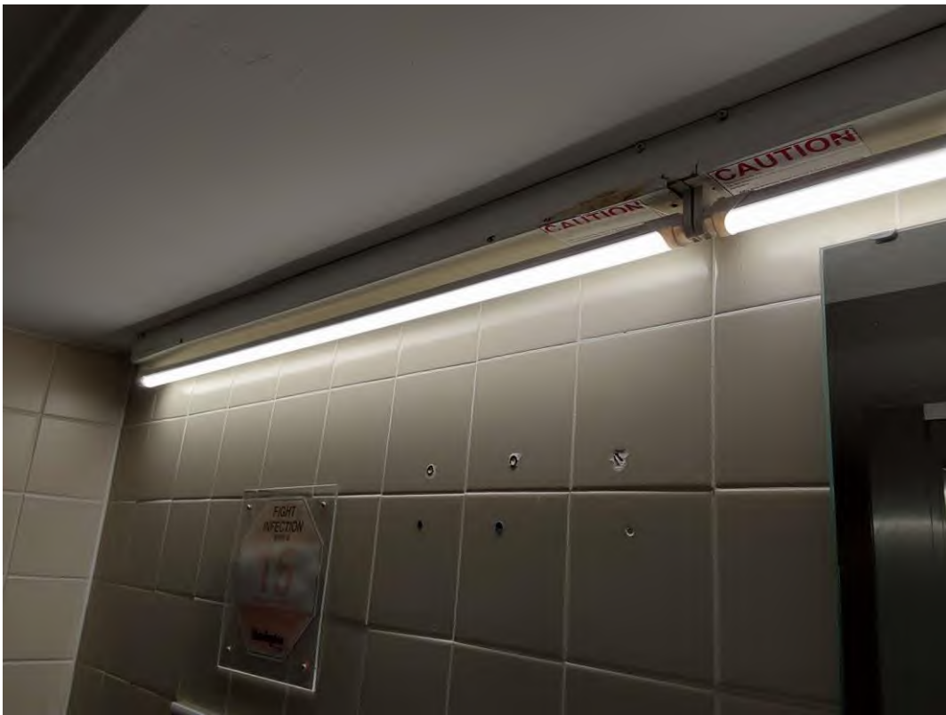
Mercury, V0000(No), LIGHT FIXTURE, LED, Men's Washroom - C2126 (Location #: 403)
