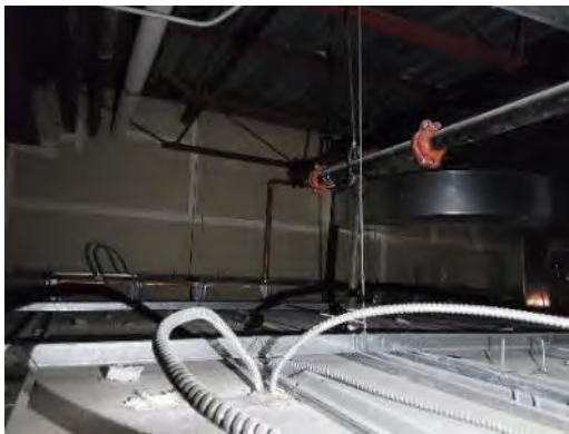
Uninsulated pipe in the Men's Washroom – B3174 (Loc. 191)
