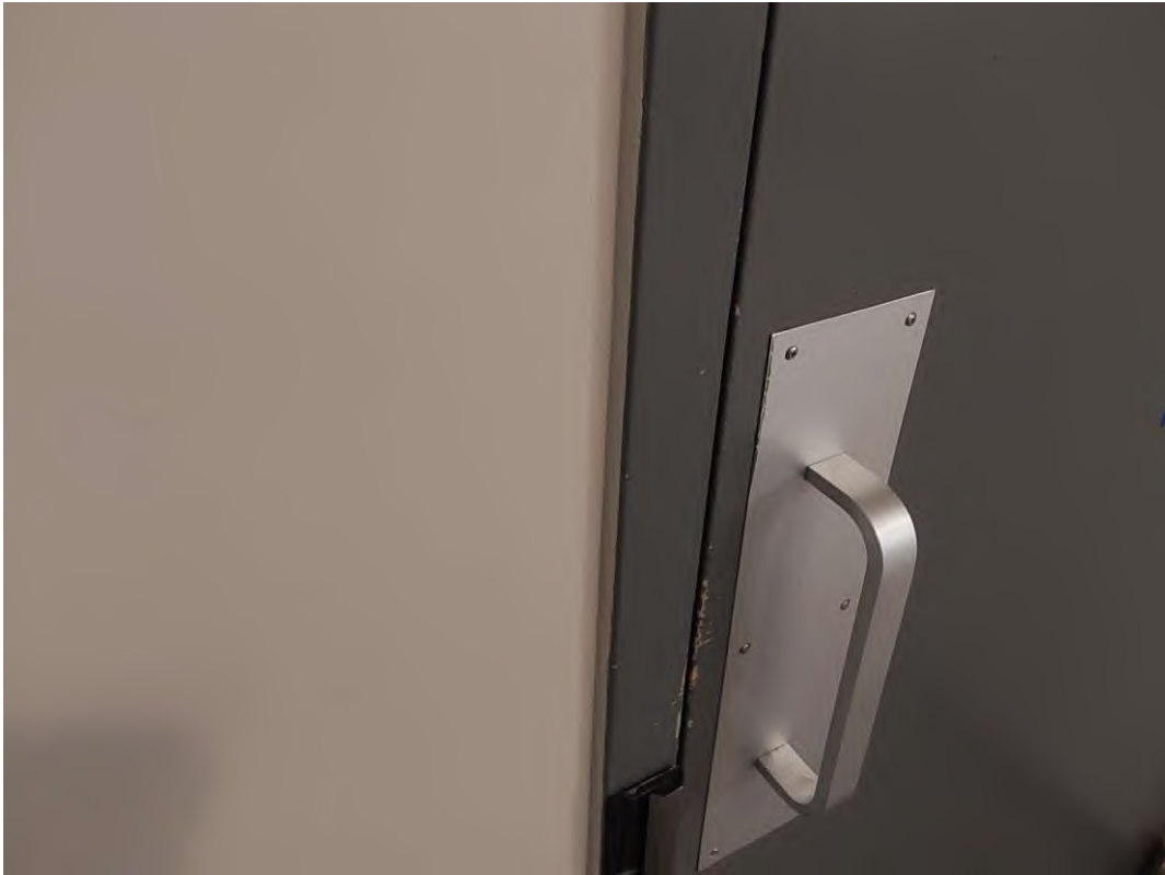
S0081C (None), Beige caulking on door frame, Wall, Caulking, Men's Washroom - B3174 (Location #: 191)
