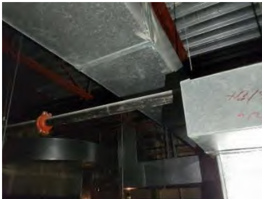
Uninsulated ducts in the Men's Washroom – B3174 (Loc. 191)
