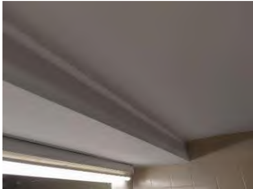
Drywall with non-asbestos joint compound on the ceiling in the Men's Washroom - C2126 (Loc. 403)
