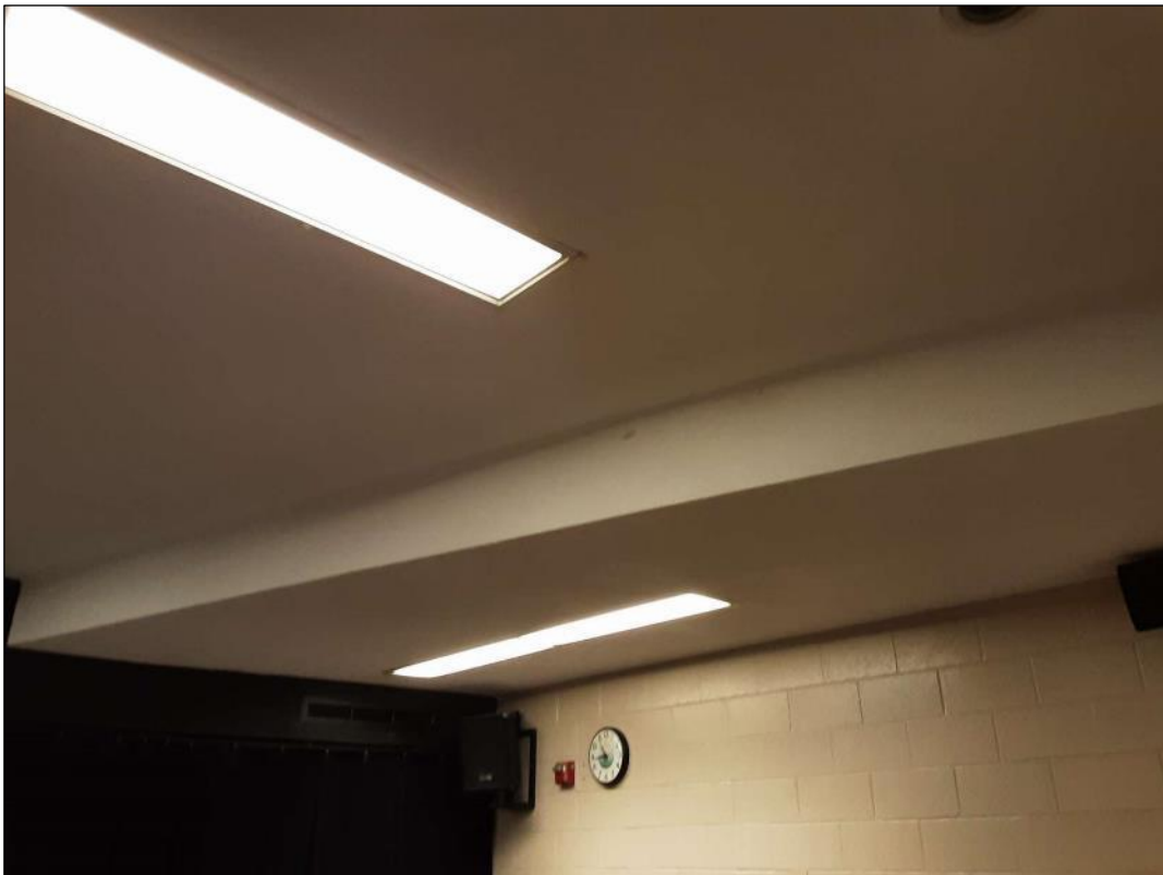
S0004A - (Confirmed Asbestos) Ceiling, Texture Coat, 102 (Location #: 1000)
