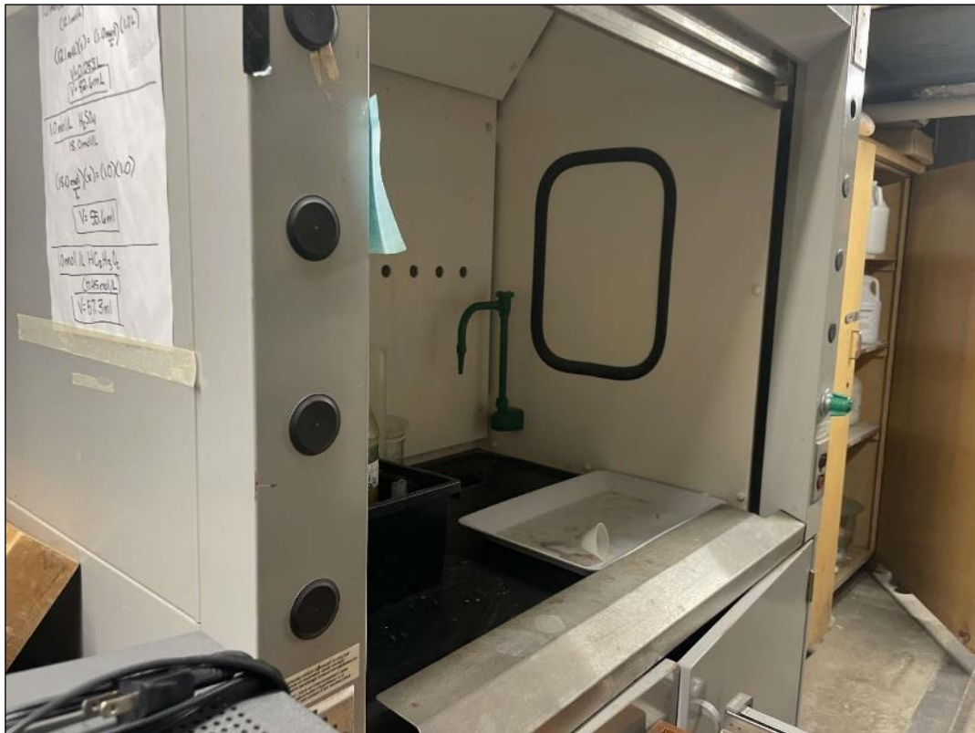
V9500 (Presumed Asbestos), Other, Fumehood, Cement Product, 238 (Location #: 2820)
