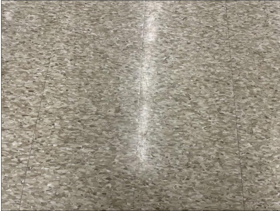
V0000 (None), 12x12 light brown with dark brown and white smears, installed post-2017, Floor, Vinyl Floor Tile and Mastic, 227 (Location #: 2360)
