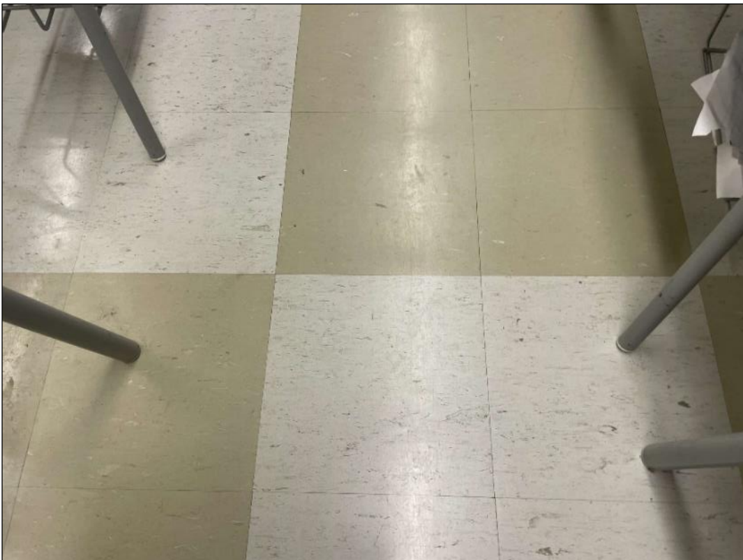
V9000 (Confirmed Asbestos), VT-5, 12x12 pale green, Floor, Vinyl Floor Tile, 205 (Location #: 2050) Previous samples ASB-125.1-3
