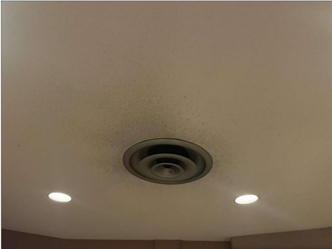
S0005A (Confirmed Asbestos), Ceiling, Texture Coat, 101 (Location #: 1610)
