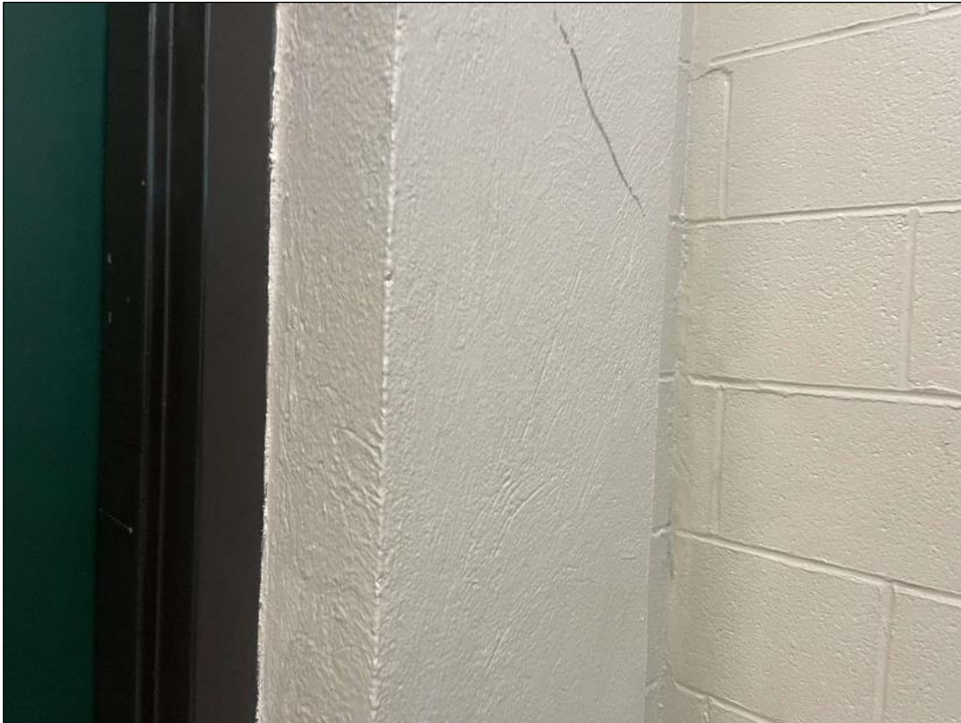
S0016A (None), Structure, Column, Paint, 233 (Location #: 2310)
