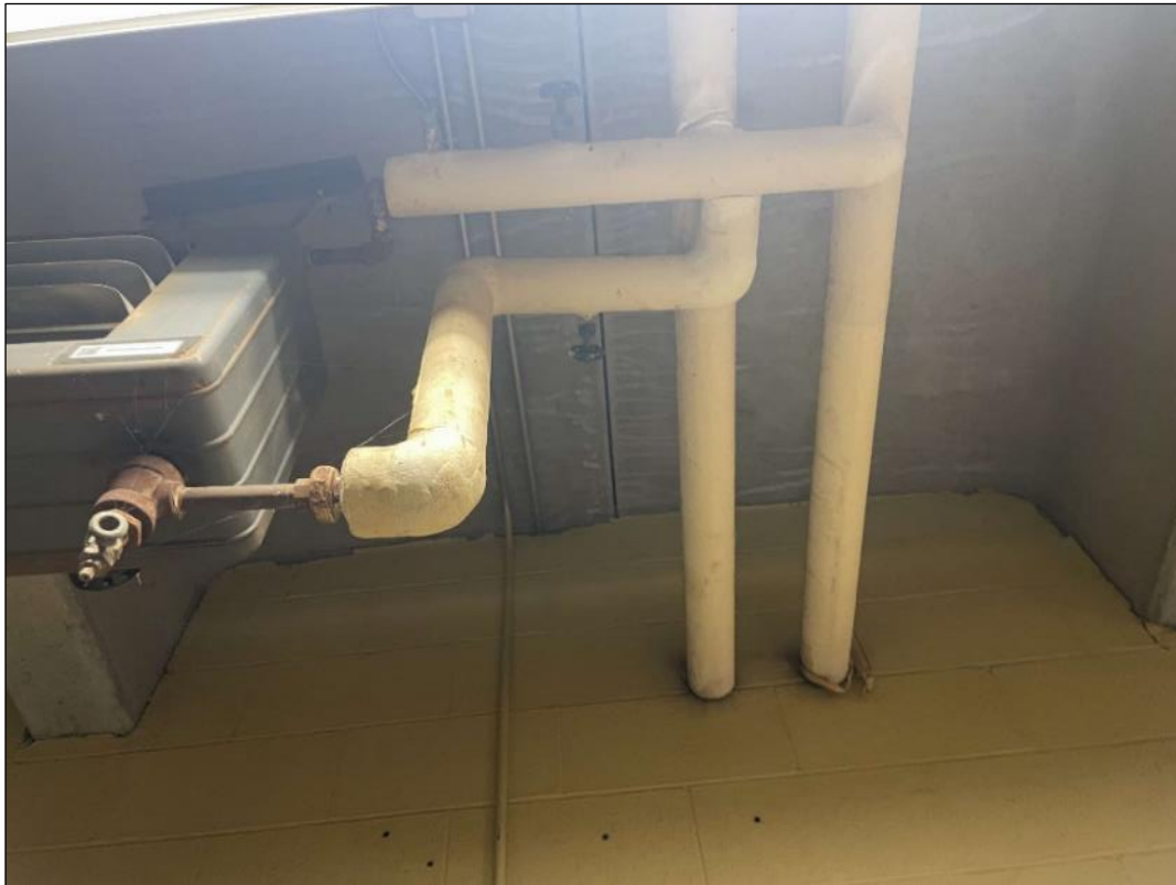
V0006 (Confirmed Asbestos), Piping, Parging Cement, 155 (Location #: 1710)
