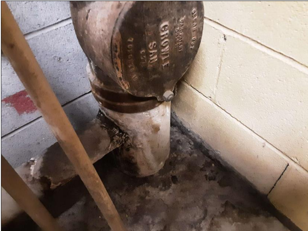
V9500 - (Presumed Asbestos), Piping, Rain Water Leader, Cement Product (Transite), 154 (Location #: 1730)
