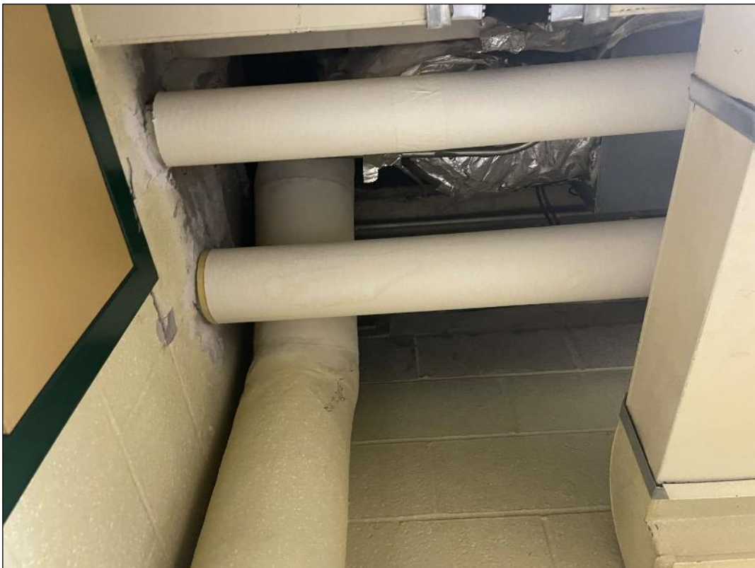
V0006 (Confirmed Asbestos), Piping, Parging Cement, 111 (Location #: 1361)
