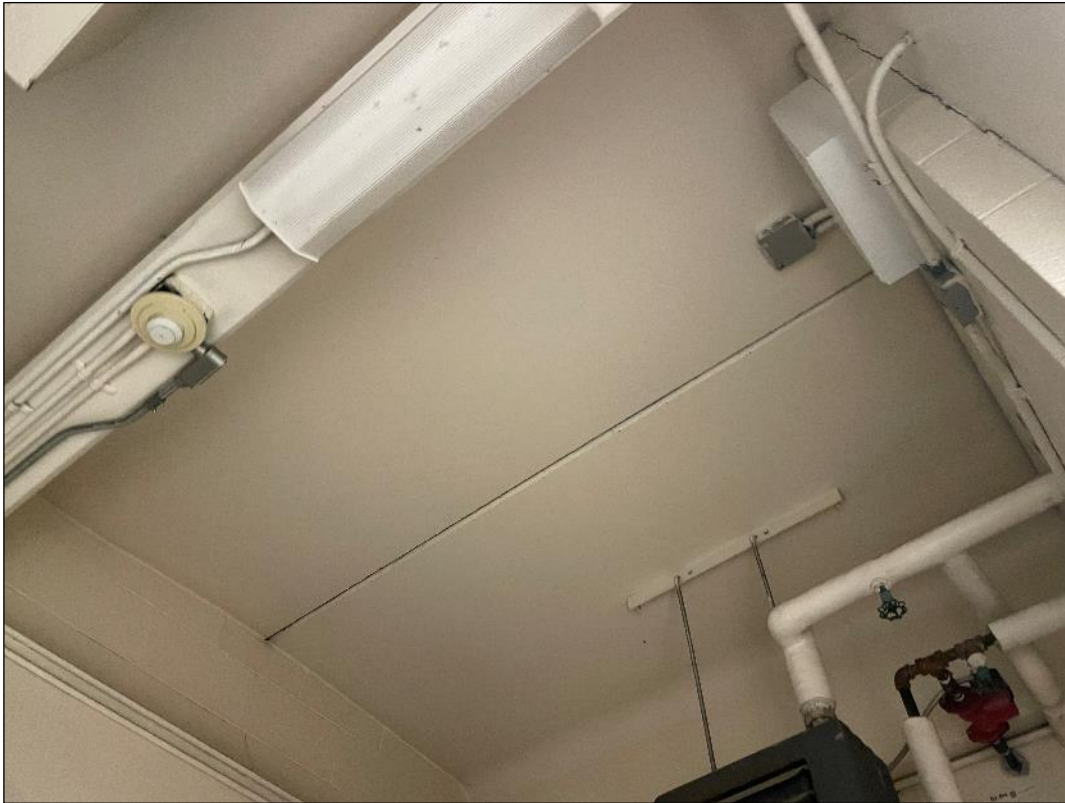
V0019 (Confirmed Asbestos), Structure, Deck, Caulking, 233 (Location #: 1772)
