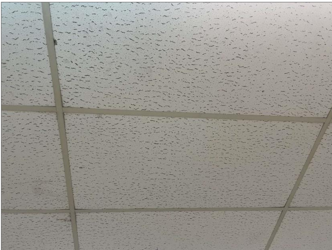
V0000 (None), 24x48 lay-in, fissures across length, Ceiling, Ceiling Tiles (lay-in), 233 (Location #: 2310) Previous samples ASB-103.1-3
