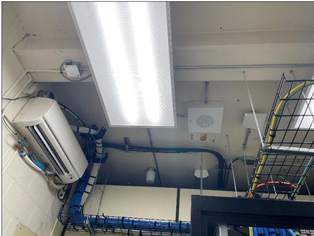
V0018 (Confirmed Asbestos), Structure, Deck, Paint, 233 (Location #: 1640)
