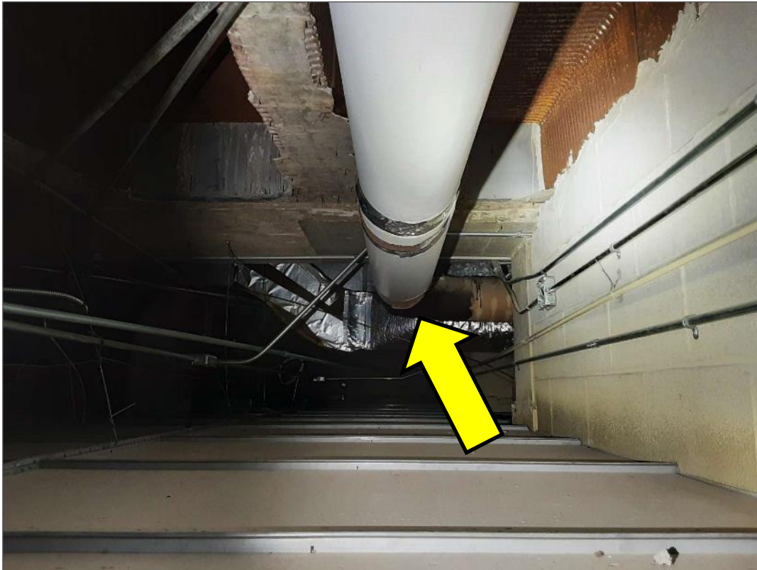
V0001 - (Confirmed Asbestos) Piping, Mastic, Over Parging Cement, 293 (Location #: 2920)
