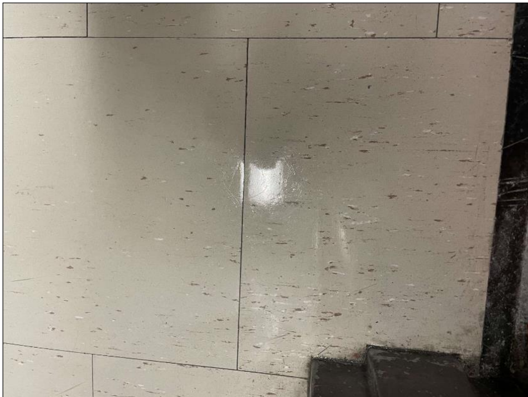
V9000 (Confirmed Asbestos), VT-9, 12x12 off-white, Floor, Vinyl Floor Tile, 223 (Location #: 2900) Historic data
