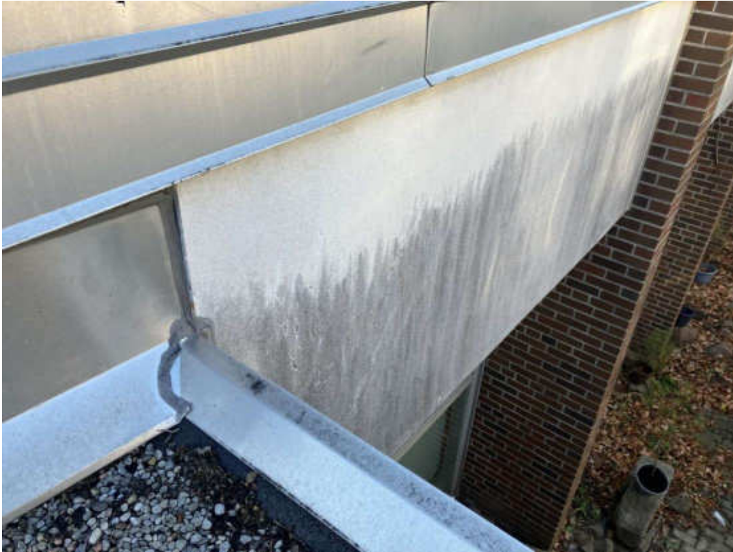
S1021A (Non-asbestos), Grey caulking on flashing, Roof E (Location #: 214) Note: adjacent to asbestos-containing cement board
