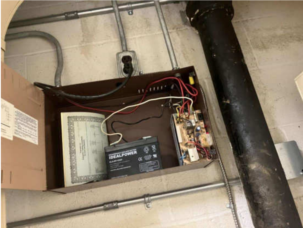
Pb (Lead) Products, V9000(Yes), Lead containing Batteries in Emer. Lights, Mechanical Room (Location #: 186)
